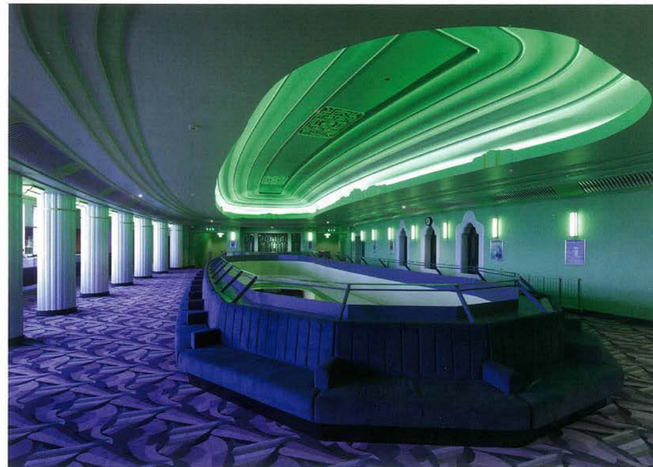
The installation also features ArcSystem MR 16 fixtures across the foyer and a DMX universe, which exceeds the normal ARC system 64 channel capability.
